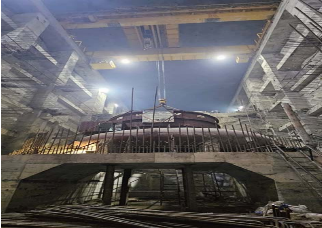
Unit-1 Pit Liner
