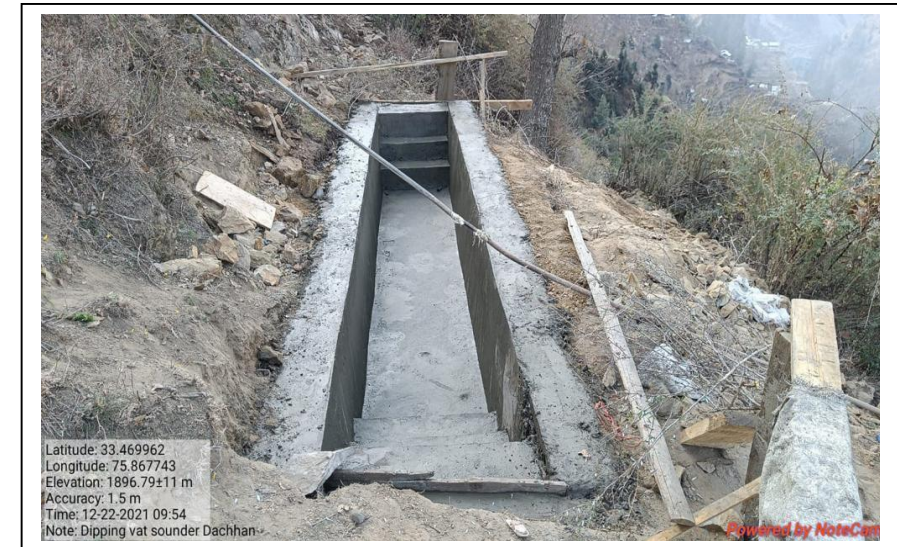
Construction of Dipping Vat at village Sounder, Dachhan, Kishtwar for sheep husbandry disease management.
