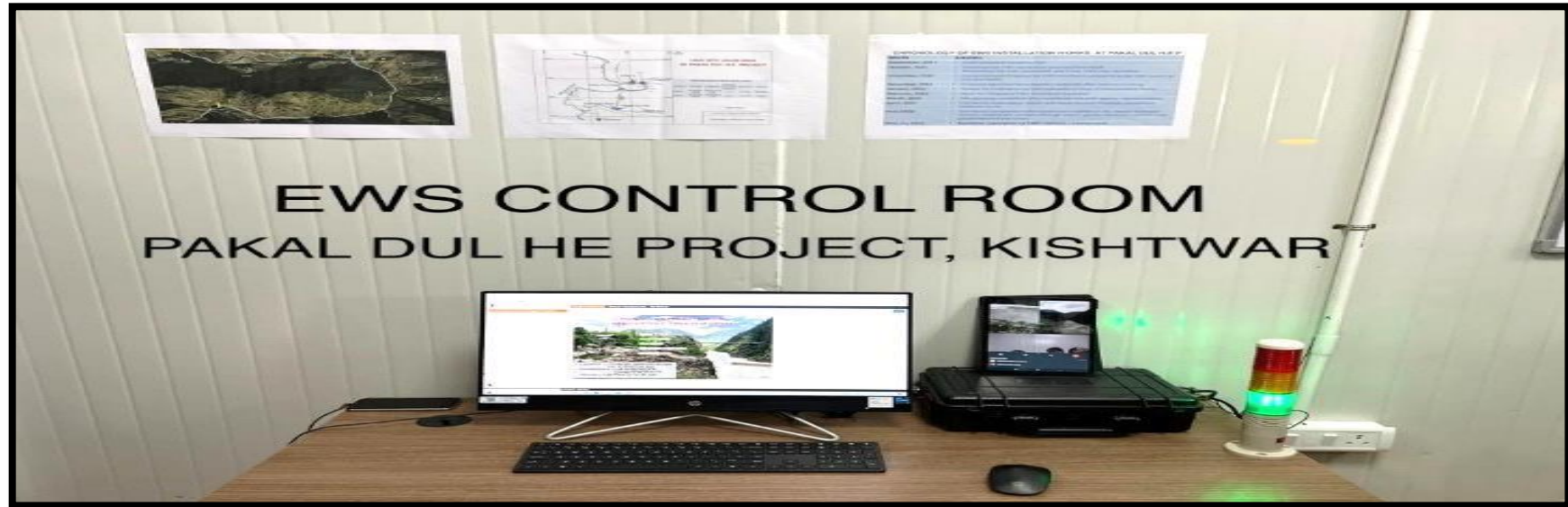
Early Warning System Control Room at Dam site of Pakal Dul HE Project
