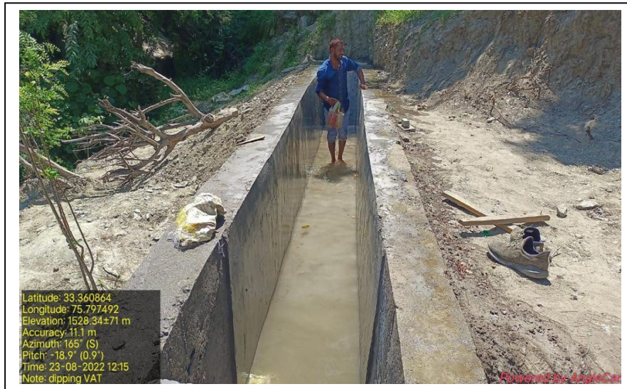
Construction of Dipping Vat at village Dool, Kishtwar for sheep husbandry disease management.
